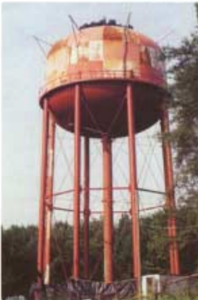
Elevated steel water storage tank at Fort Meade had 8900 sq ft of lead-based paint removed with the blast media additive.
